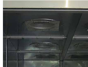
Large internal fans
